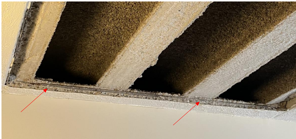
Figure 3: Edge of soffit at failure line (note reinforcing steel)
