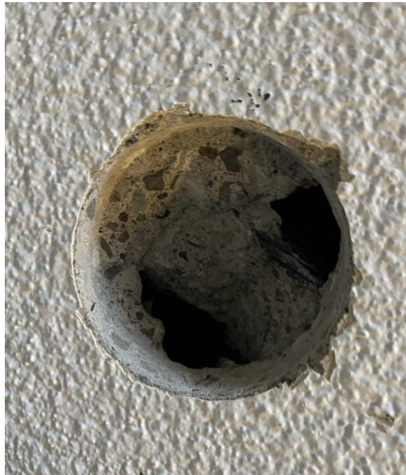
Figure 4: Core sample at adjacent panel to the failed panel in Unit 19
