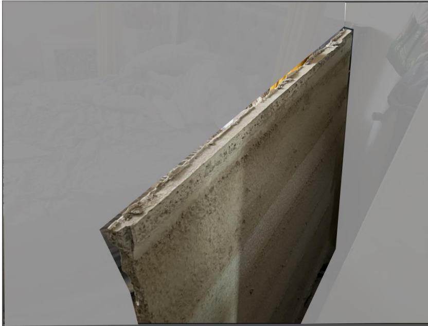
Figure 1: Section of Panel that fell
