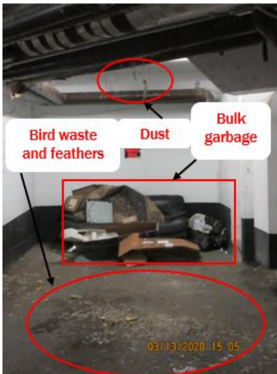
Photograph 5: Underground garage not properly cleaned
