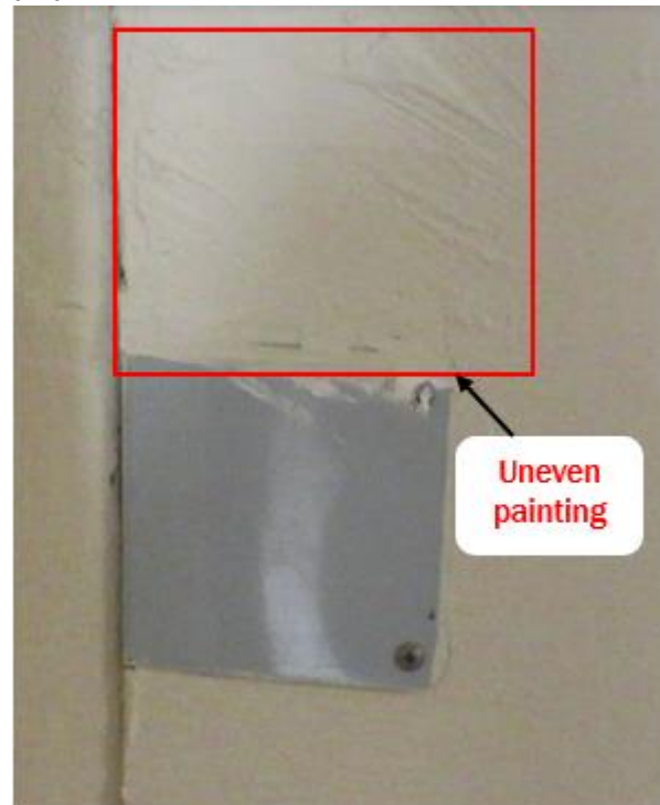
Photograph 4: Uneven painting on unit door
