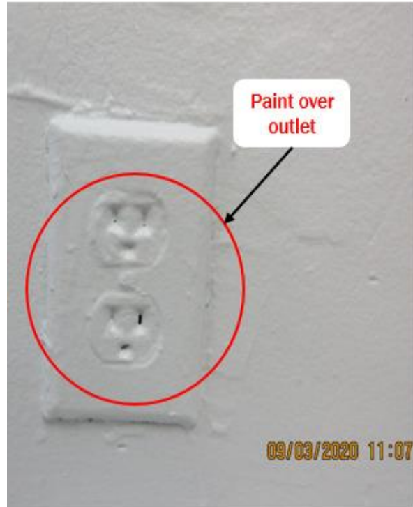
Photograph 2: Paint over electrical outlet at vacant unit
